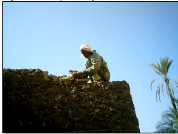
Figure 19: One of the Workers Laying Karshif Blocks to Form a Wall. Taken by the researcher.
